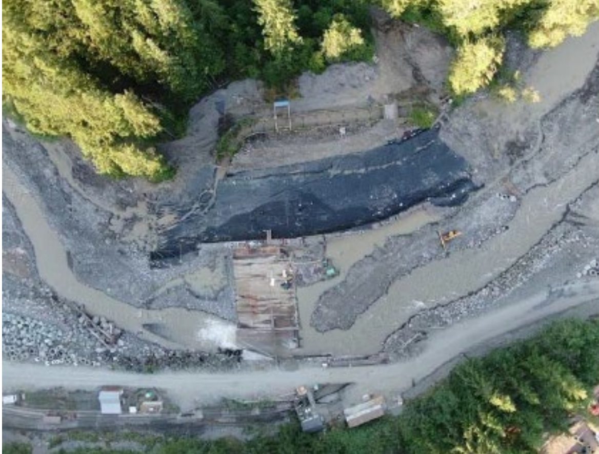
A photograph of the liner prior to diverting flows to the right bank - July 27, 2020. This photograph was included in a report prepared by Shane Cherry Consulting.
