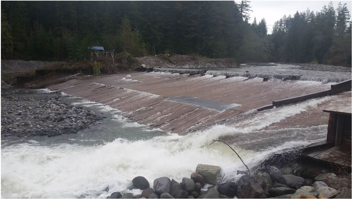
Electron Dam, prior to the commencement of construction in the summer of 2020. Electron submitted this photograph to Pierce County as Part of their Phase I Engineering Design Report, dated February 2017. [Overlay text removed]
